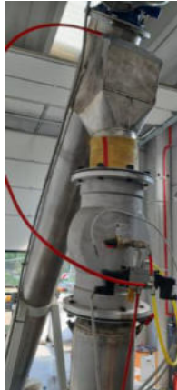
Figura 13: By pass valvole pneumatiche
